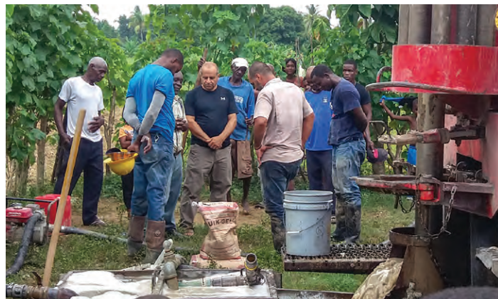
Charlie DeTellis leads a time of prayer with the well drillers at the New Missions church and school in Flon, Haiti.
