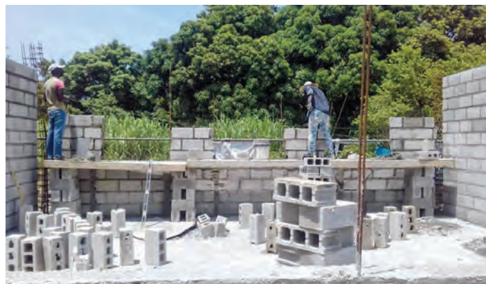
A new church is under construction on our campus in Flon, Haiti. This is built 100% by Haitians—providing jobs to support their families.
